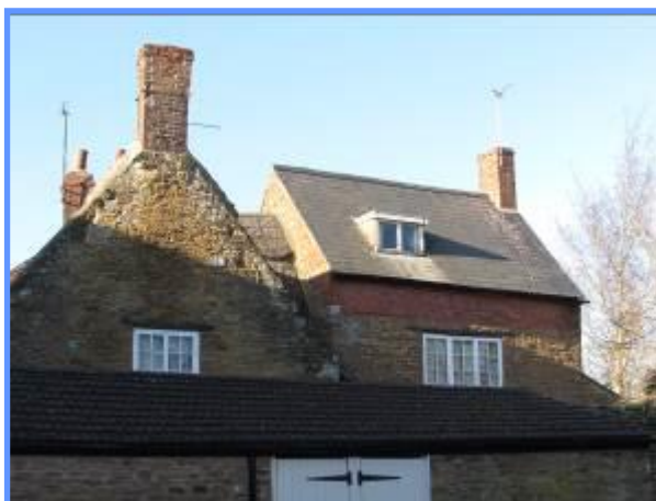
Figure 39 Mixed ridgelines and roofing materials are sometimes found on the same historic property. Here the new gable is in keeping, and appropriately not thatched.
