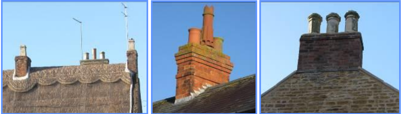
Figure 45 An example of a brick chimney stack in the village, with multiple chimney pots. This is characteristic of larger properties.
